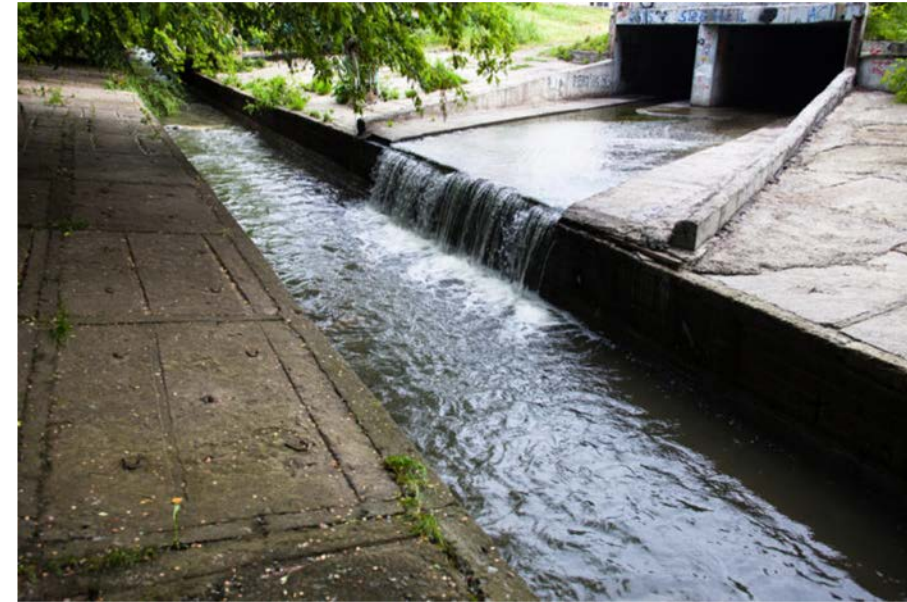
A typical open stormwater drain. Sydney, Australia
